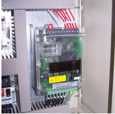
fig. 3.6.6 R&M's standard VFD Control located inside the bridge control panel.
